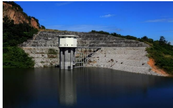
Figure 4 – A View of Draw-off Tower
