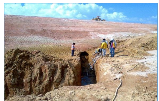
Figure 7 - Concentrated Leak at left abutment of existing dam
