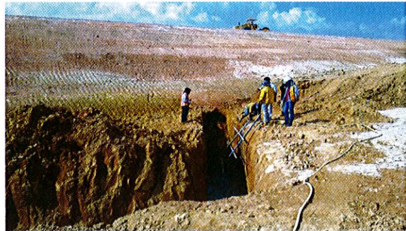
Figure 9 - Concentrated Leak at left abutment of existing dam
